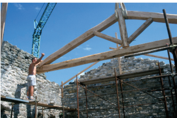
Fig. 4. Positioning the first truss of the medieval wing on the original stone brackets. Image by the author.
