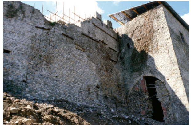
Fig. 3. The same wall seen from the outside after the re-integration of the large loss in the masonry that made the wall unstable. Image by the author.
