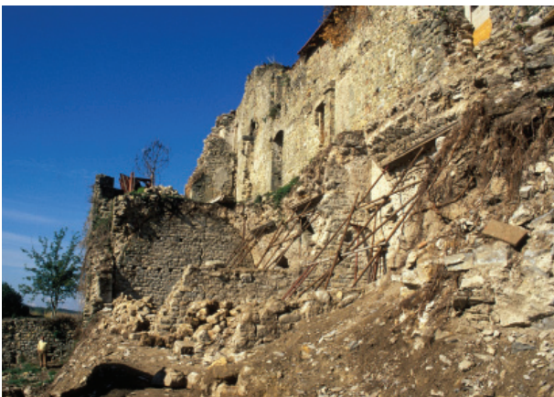
Fig. 9. The main room of the south wing: on the right hand side it is visible the springing of the collapsed vault whose geometry can be easily followed on the transverse wall at the bottom. On the left, above the escarpment, the base of the south wall. Image by the author.
