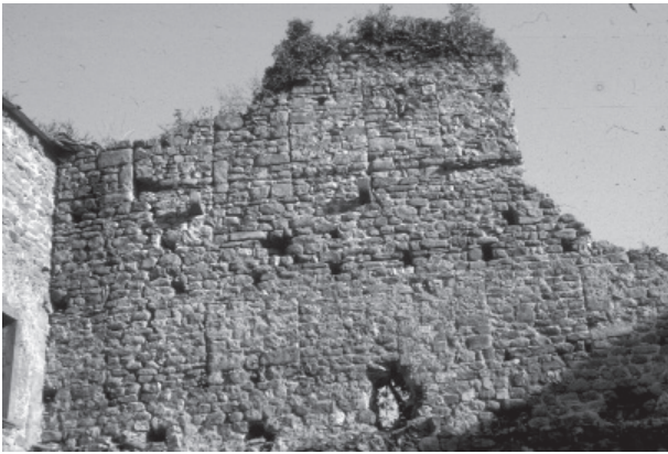
Fig. 2. The enceinte wall seen from the inside: on this beautiful raking light one can see, just below the top portion of the masonry, two dovetail merlons and, under the line of putlogs, the remains of an older square crenellation. Image by the author.
