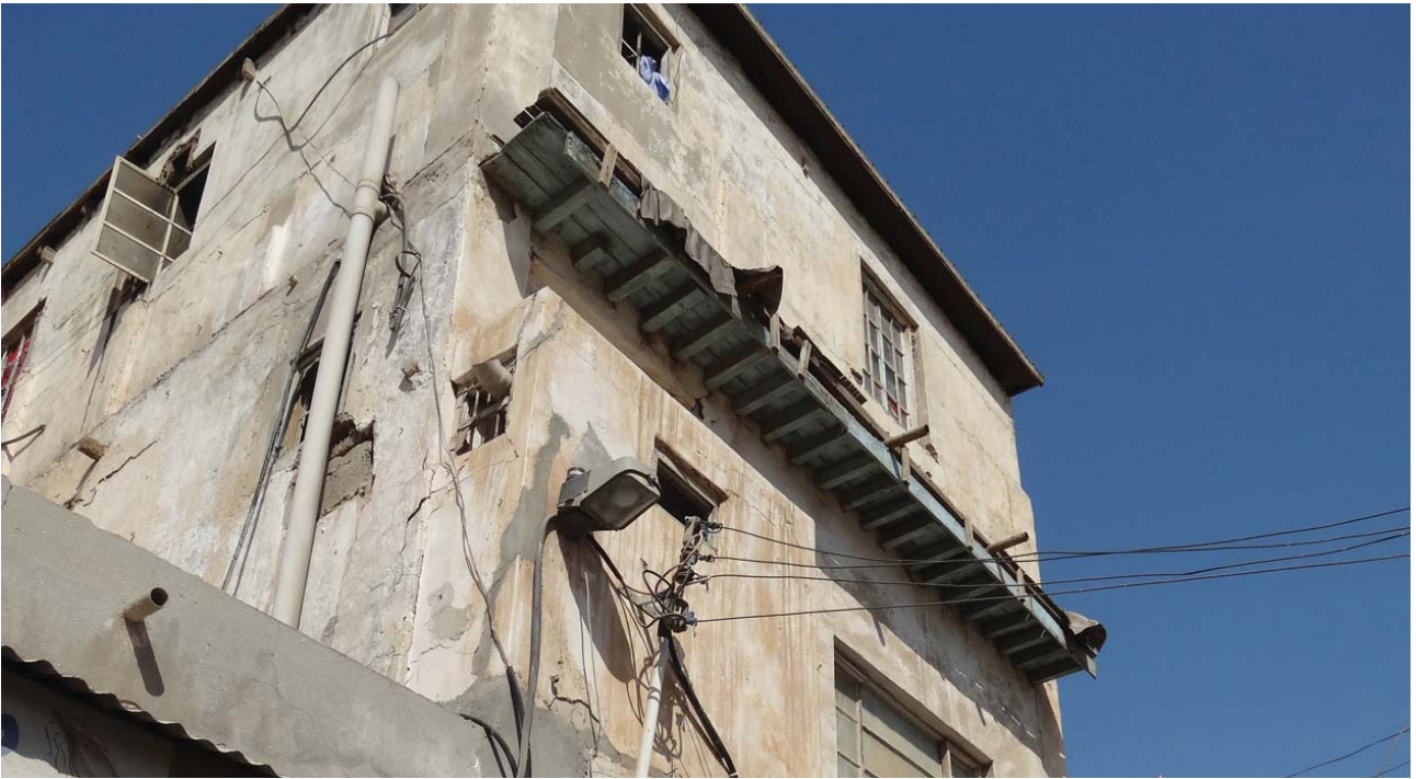
Fig. 12. Square beams extending to create a shading elements on the façade in a similar way to the traditional danshal beams. Image by Bahrain Authority for Culture and Antiquities.
