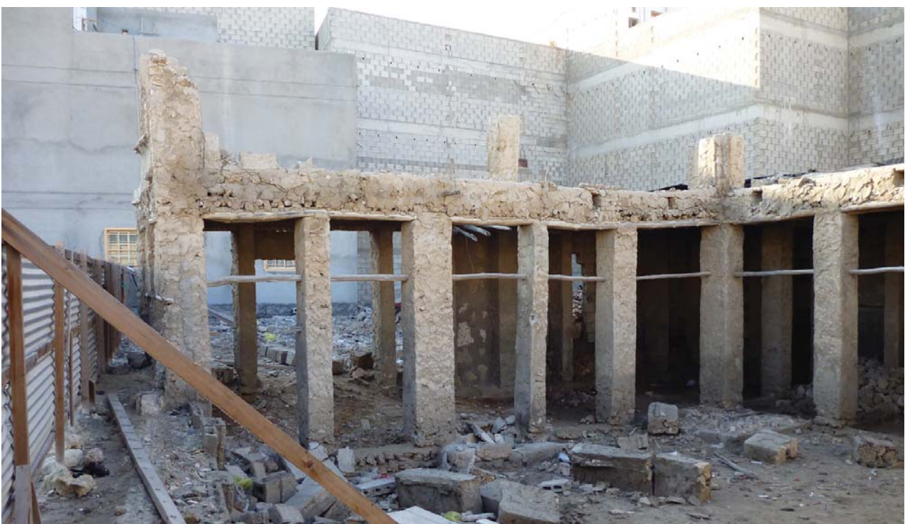
Fig. 10. Basic traditional structural system used for warehouses. Image by Bahrain Authority for Culture and Antiquities.
