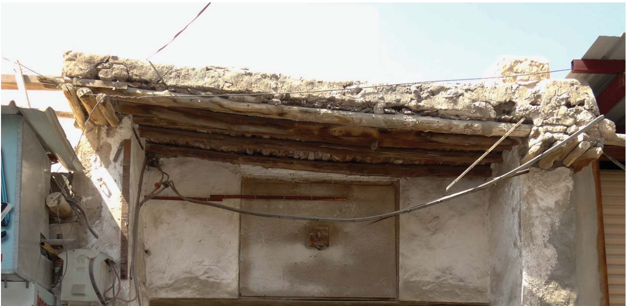
Fig. 9. Shading element on a shop's façade clearly showing the traditional ceiling system. Image by Bahrain Authority for Culture and Antiquities.
