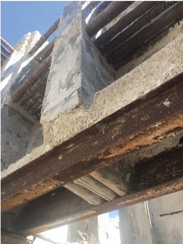
Fig. 7. Steel beam system replacing the traditional danshal beams to enable wider openings. Image by Bahrain Authority for Culture and Antiquities.
