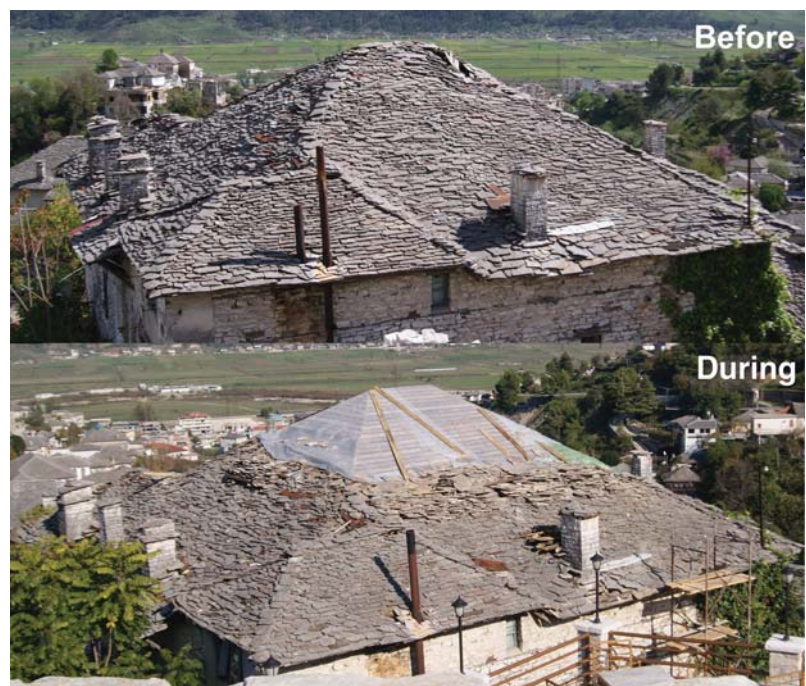
Fig. 8. Two photos of Gurgai house show the hole in the roof and repair works underway to restore it. Images by CHwB.
