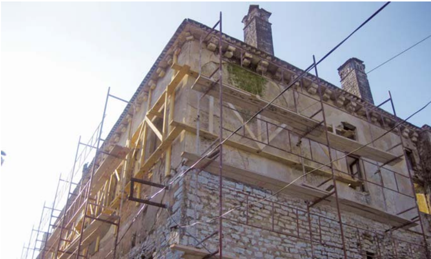
Fig. 7. A view of Hadëri house (left) shows support structures that shore up the remaining walls. Image by CHwB.
