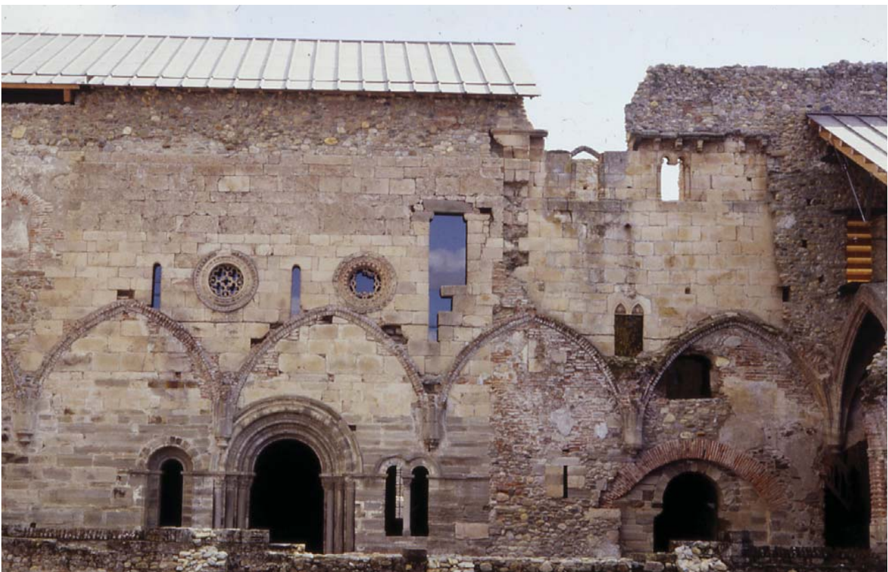
Fig. 5. Wall with traces from different historic stages. Monastery of Santa María de Carracedo, León, Spain. Restoration project by Susana Mora and Salvador Pérez Arroyo.
